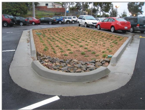
Figure 7: Bioretention within parking lot.
