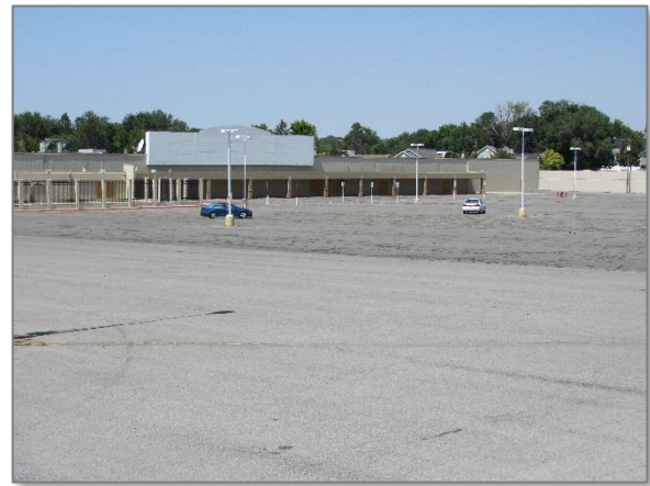
Figure 1: Impervious parking lot with no pervious areas or storm water quality features.
