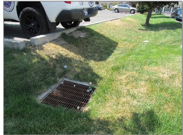
Figure 3: Curb cut at downstream end of parking lot.
