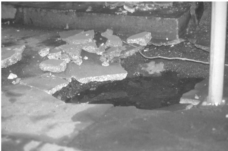
Figure 1-19. This basement floor broke from hydrostatic pressure
